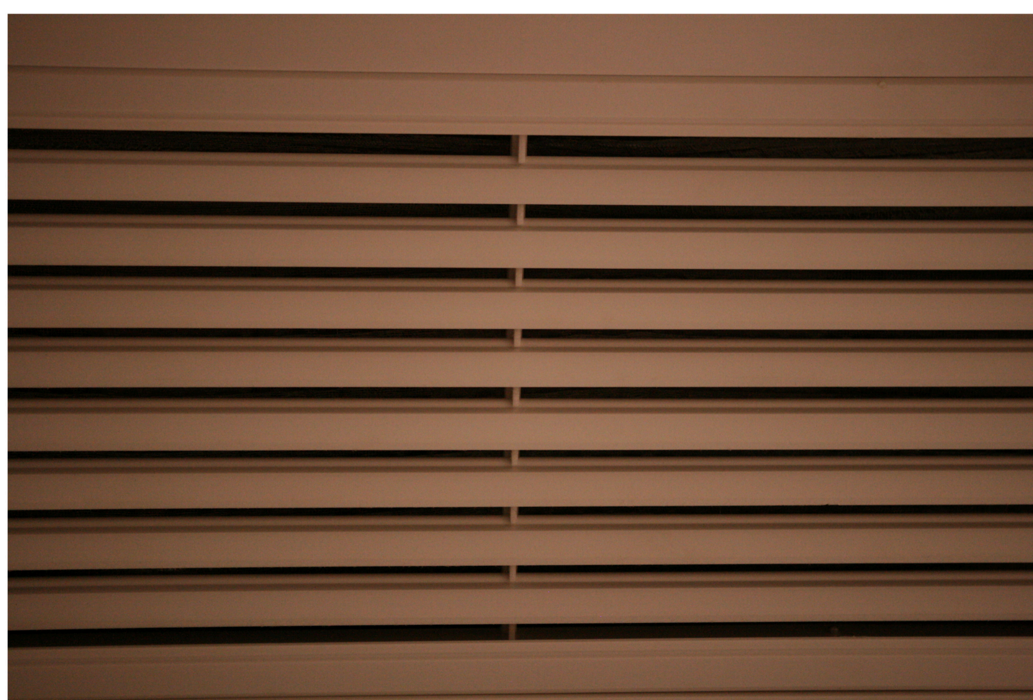
The folds of an air conditioner. The photo shows horizontal lines that form patterns
